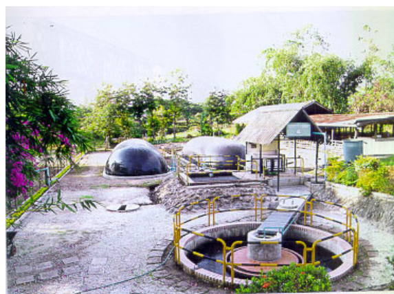
Circulation tank and biogas domes at pig farm (Pak Tho District, Thailand)
